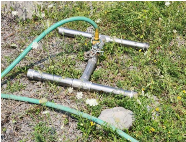
Figure 4 Coarse Bubble Aerator
